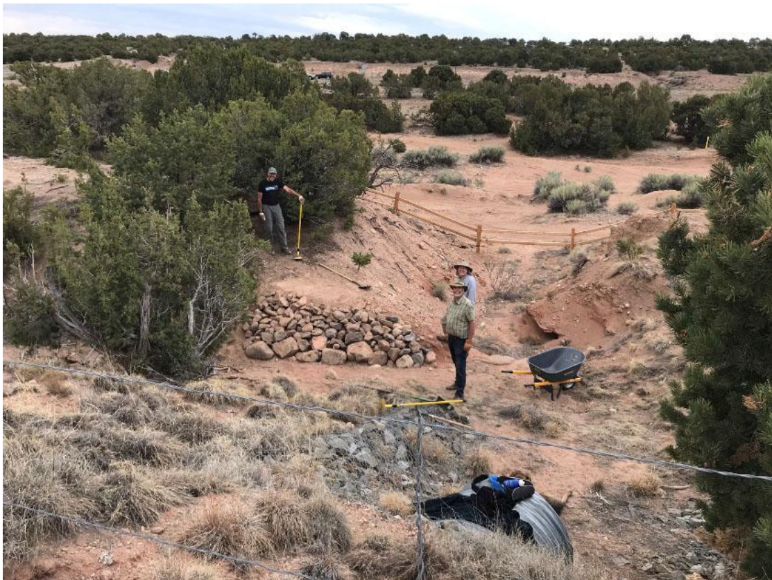
2020 grant recipient Santa Fe Conservation Trust. La Tierra Chili Line Trail - volunteers complete a retaining wall to support one side of a wooden footbridge (May 2021).
